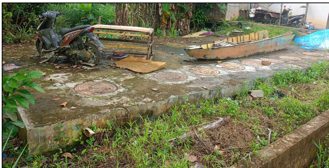
Fig 2. Location and Condition of the Tura Tea Wastewater Treatment Plant in Palaran District, Handil Bakti Village
